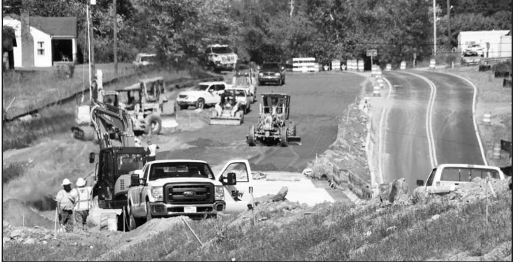
Construction continues on the new bridge replacing the old Brasstown Creek Bridge, which has been in place since 1940. Photo by Shawn Jarrard
